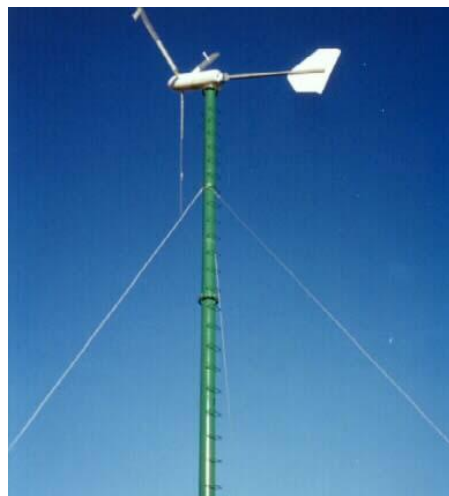
Figure 4.4. Solener Velter XV 15-kW turbine
