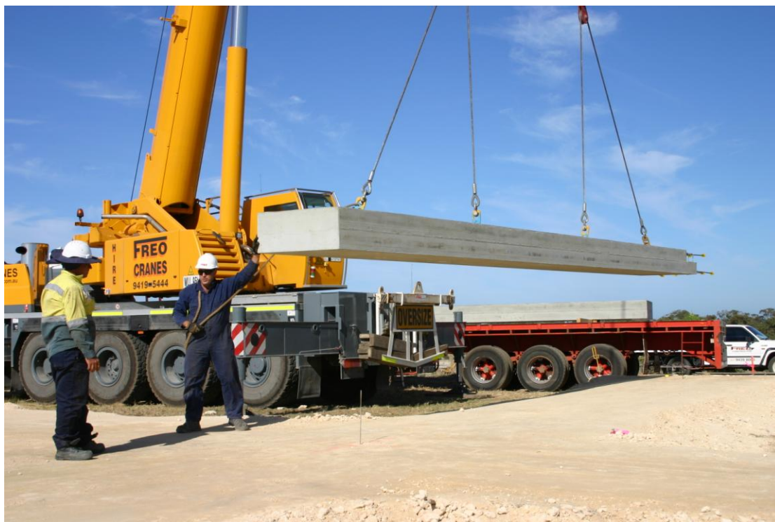
Figure 2.6. Construction of the testing facility for the National Small Wind Turbine Centre
