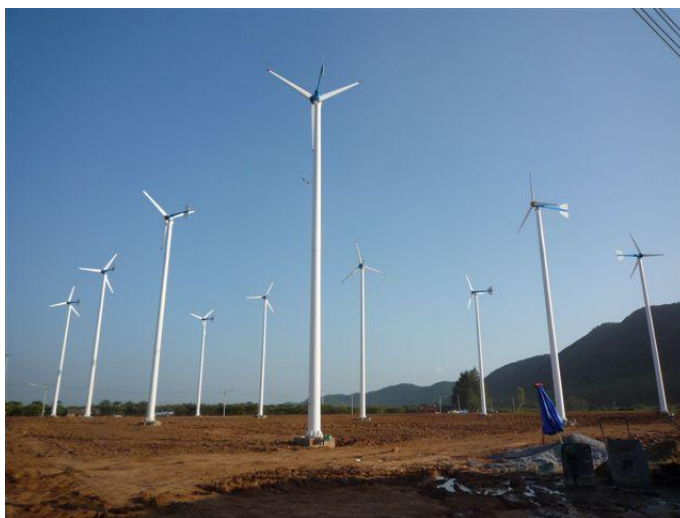
Figure 3.2. SAMDORIE installed in Thailand
